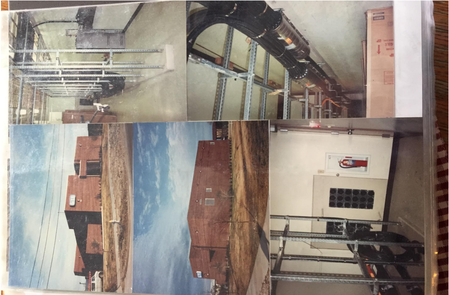
Complex & technical GTE Exchange Building in Flower Mound, TX. I was Project Manager for complete design, construction documents & Construction. Completed all documents & details, managed construction.
